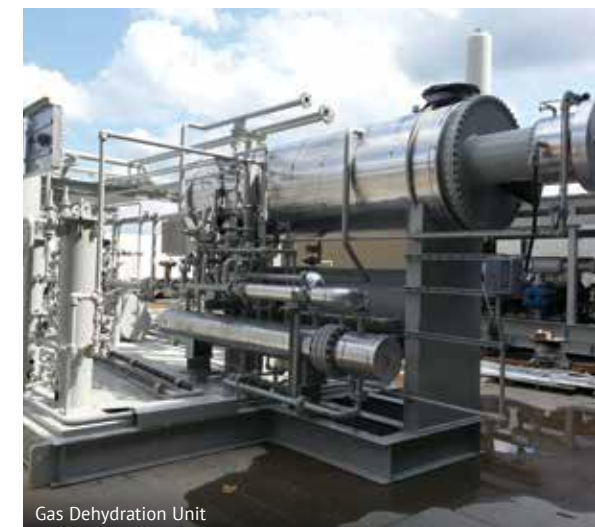
Gas Dehydration Unit
