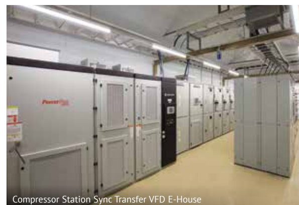
Compressor Station Sync Transfer VFD E-House
