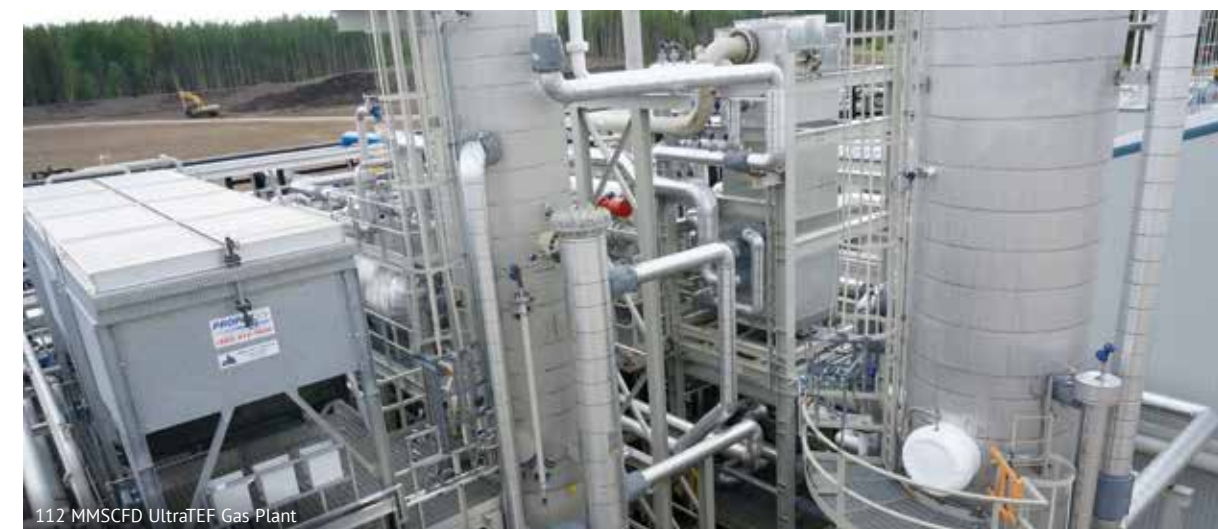
112 MMSCFD UltraTEF Gas Plant
