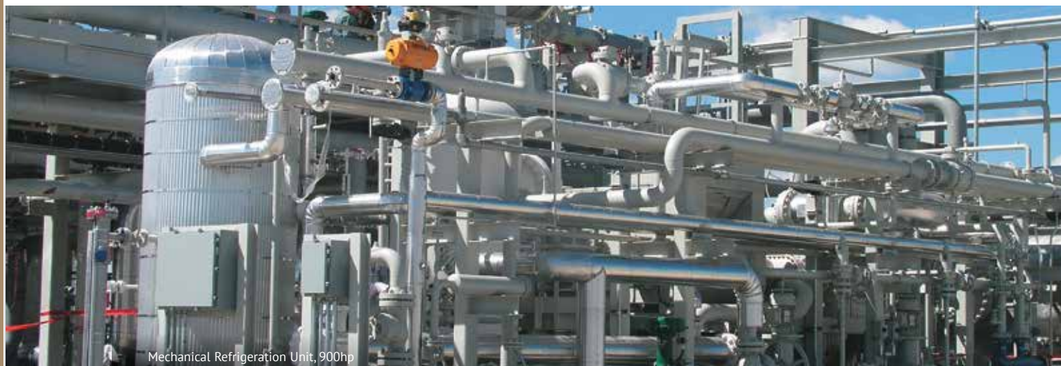
Mechanical Refrigeration Unit, 900hp
