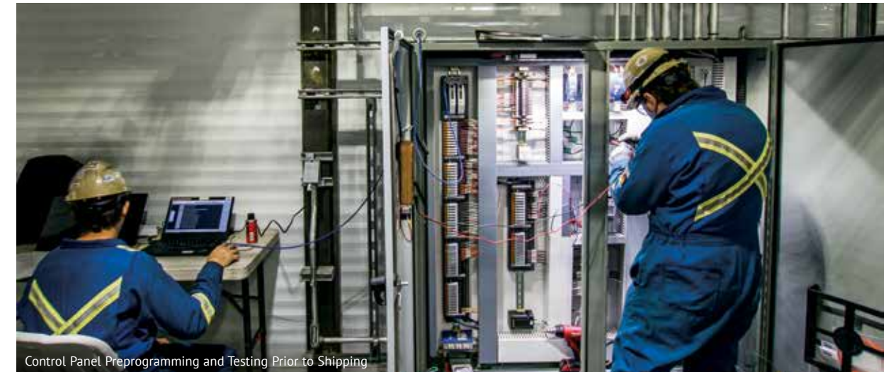
Control Panel Preprogramming and Testing Prior to Shipping
