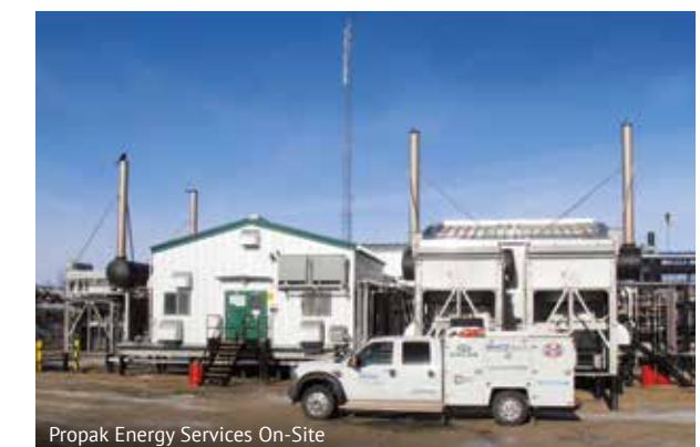
Propak Energy Services On-Site
