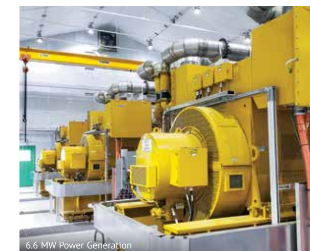
6.6 MW Power Generation
