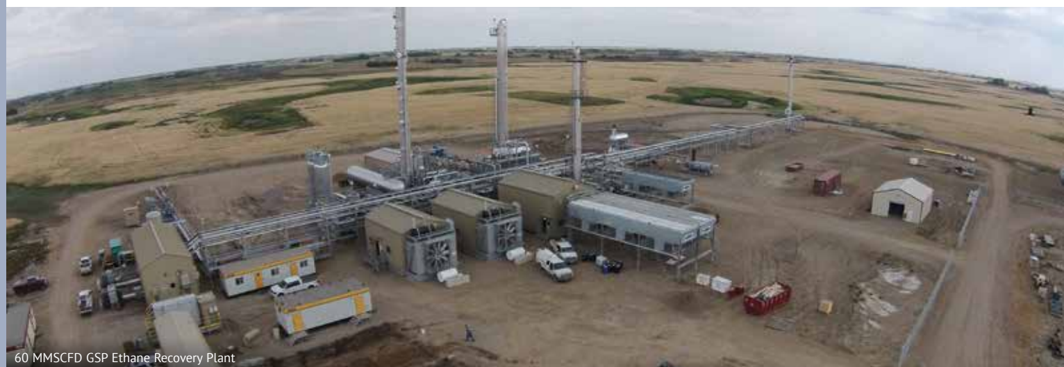
60 MMSCFD GSP Ethane Recovery Plant
