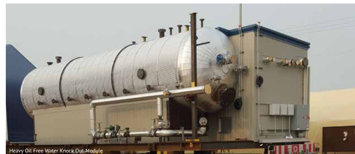
Heavy Oil Free Water Knock Out Module
