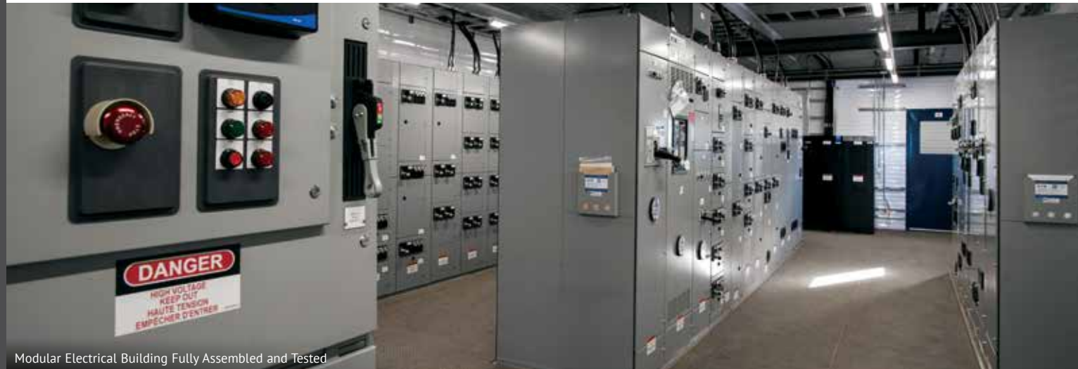
Modular Electrical Building Fully Assembled and Tested
