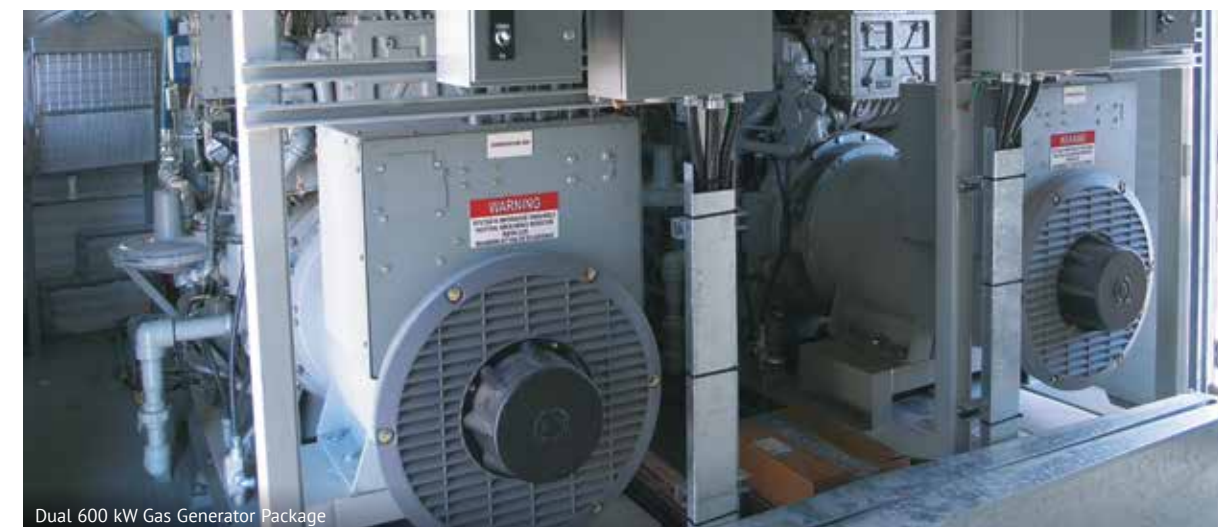
Dual 600 kW Gas Generator Package
