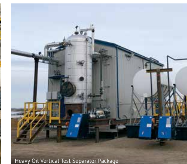
Heavy Oil Vertical Test Separator Package
