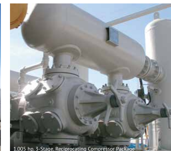
1,005 hp, 3-Stage, Reciprocating Compressor Package
